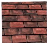
Handmade clay plain tiles to plots 1, 2 and 3 main dwelling roof areas, and roof area of cart-lodge serving plot 3.
